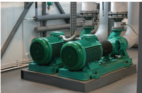
HVAC, pumps and valves.
