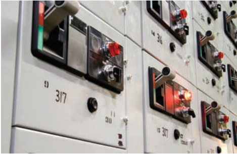
Power generation and distribution.
